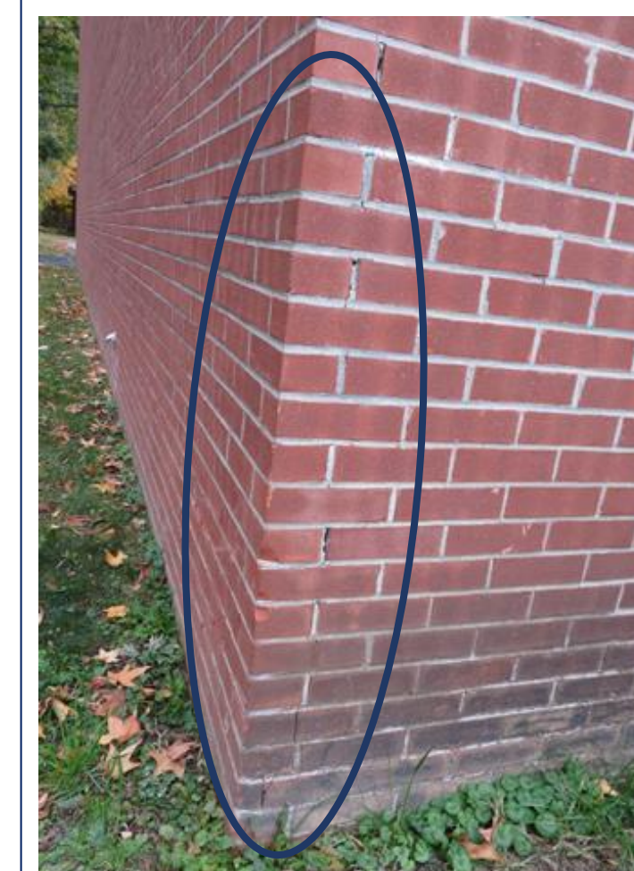
Figure 7: Exterior Wall Step Cracking
