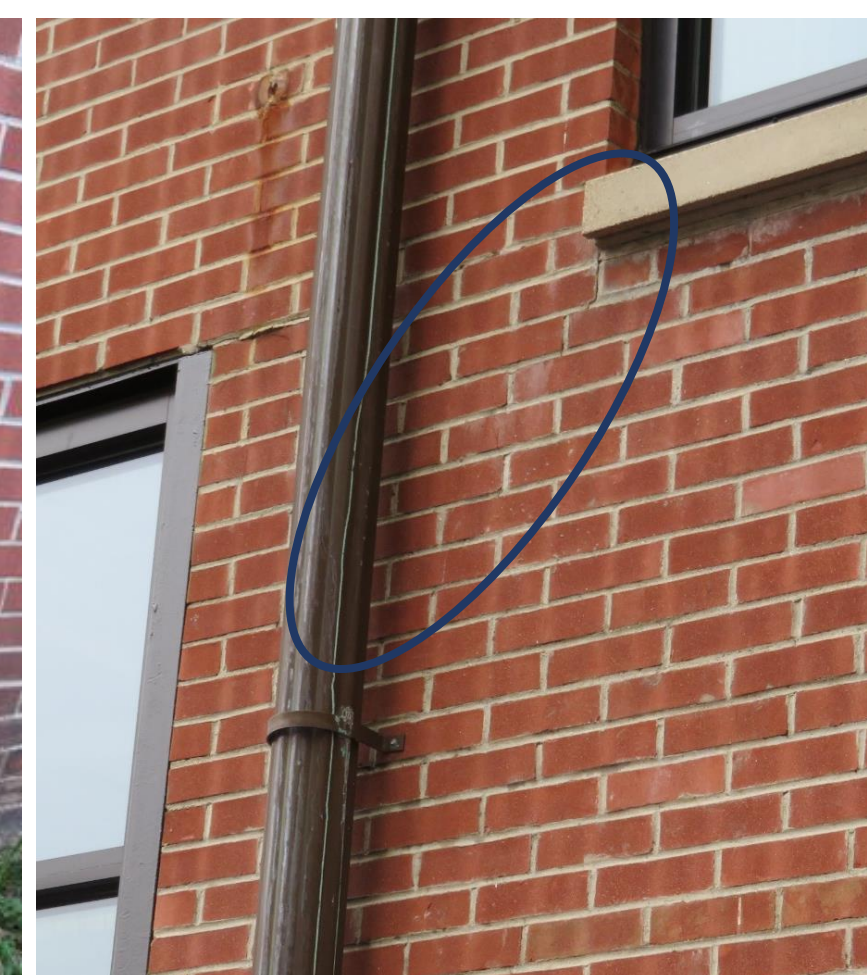
Figure 8: Exterior Step Cracking by Window Along East Wall
