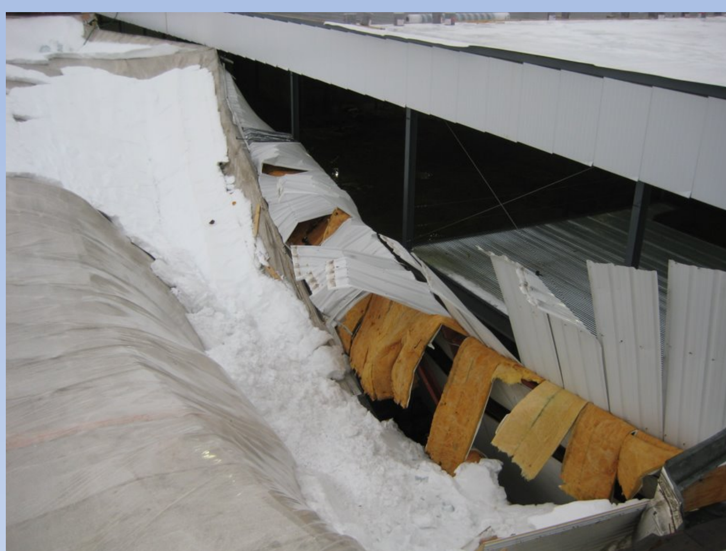
Figure 5: North View of Collapse
