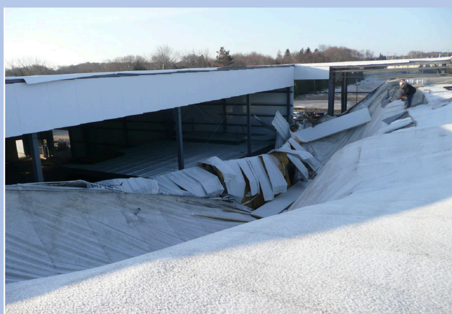
Figure 2: South View of Collapse
