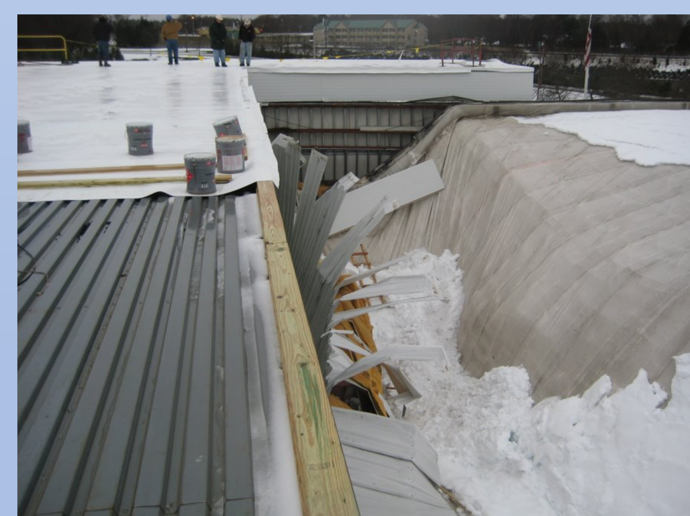
Figure 3: South View of Collapse
