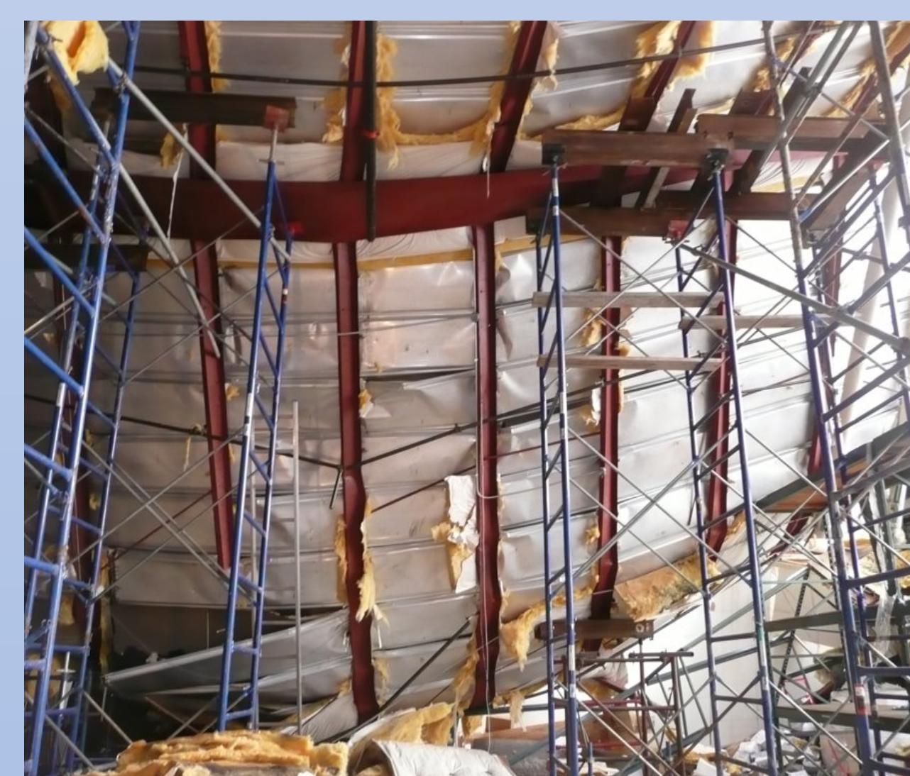
Figure 4: Interior View of Collapse
