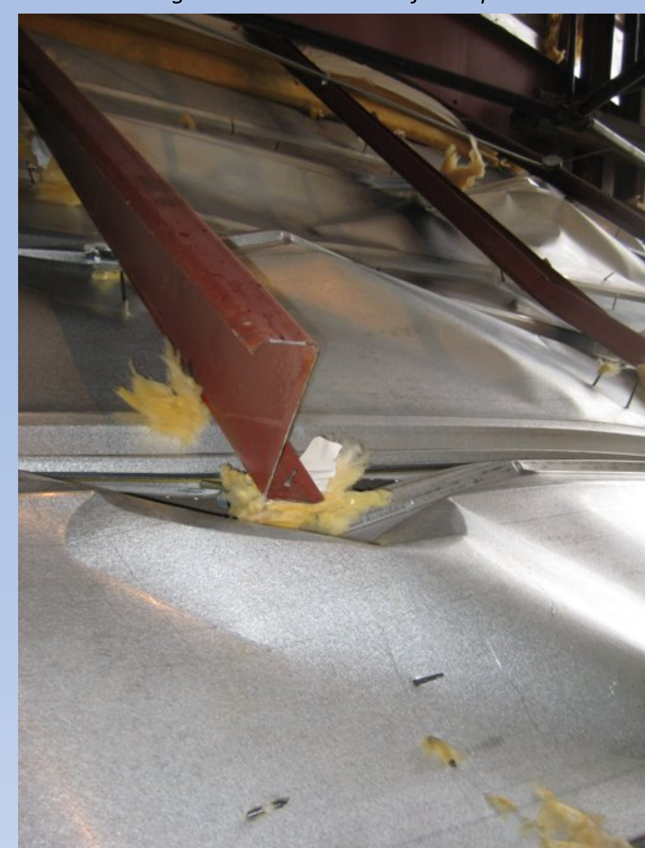
Figure 7: Faulty Purlin Splice
