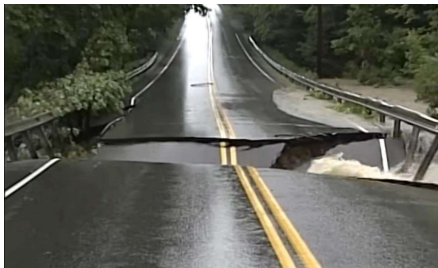
Fig. 1: Culvert failure during large flood in Freeport, Maine, in August 2008
