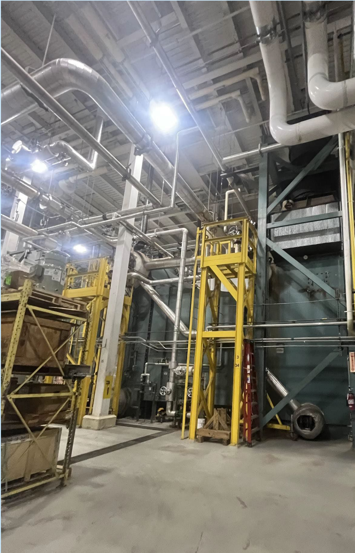
Left: Photo of inside the power plant
