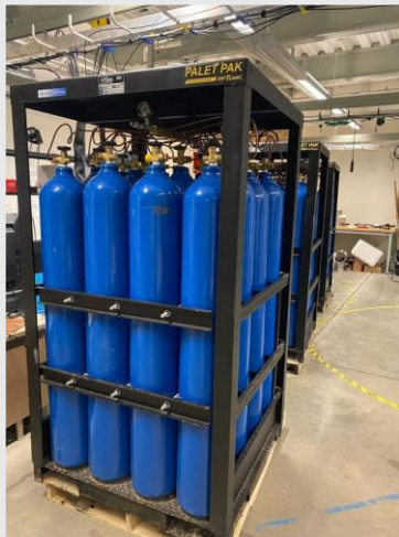
HP Gas Cylinders
