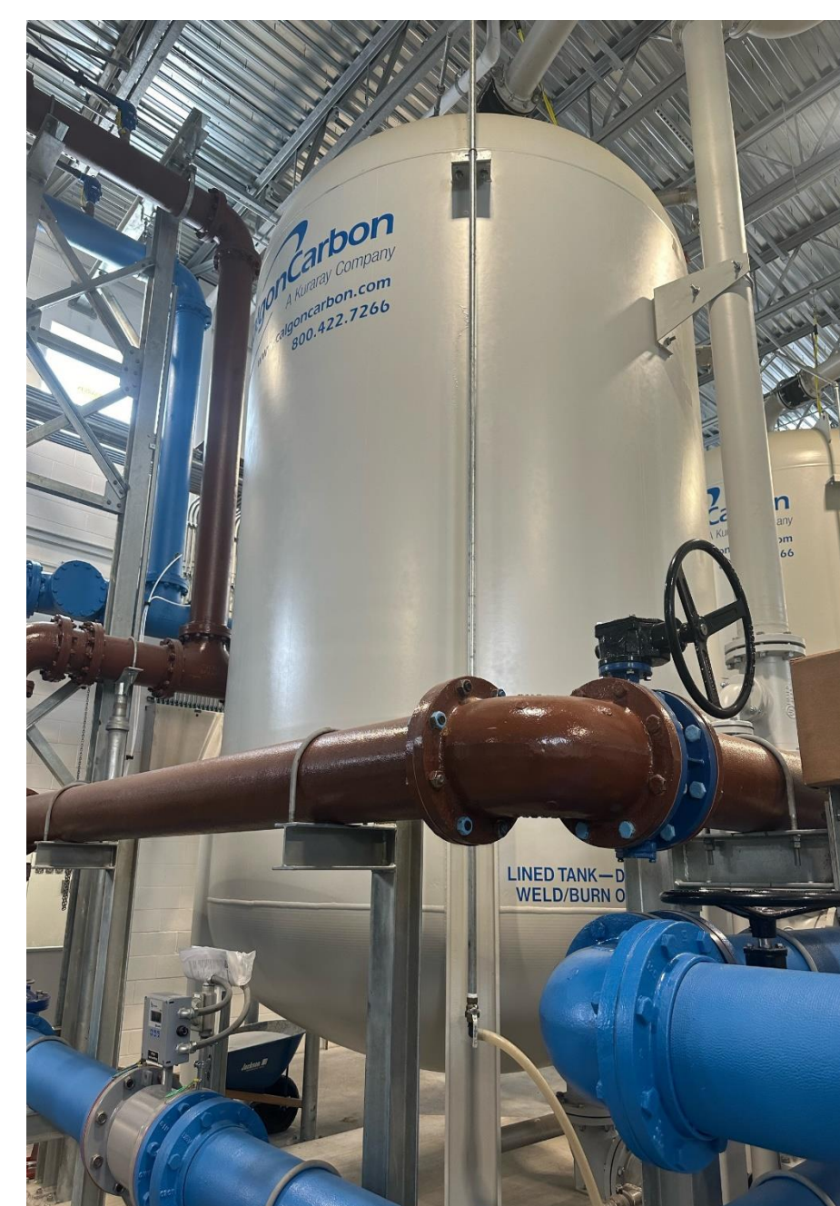
Fig. #4: Calgon Activated Carbon Contactor
