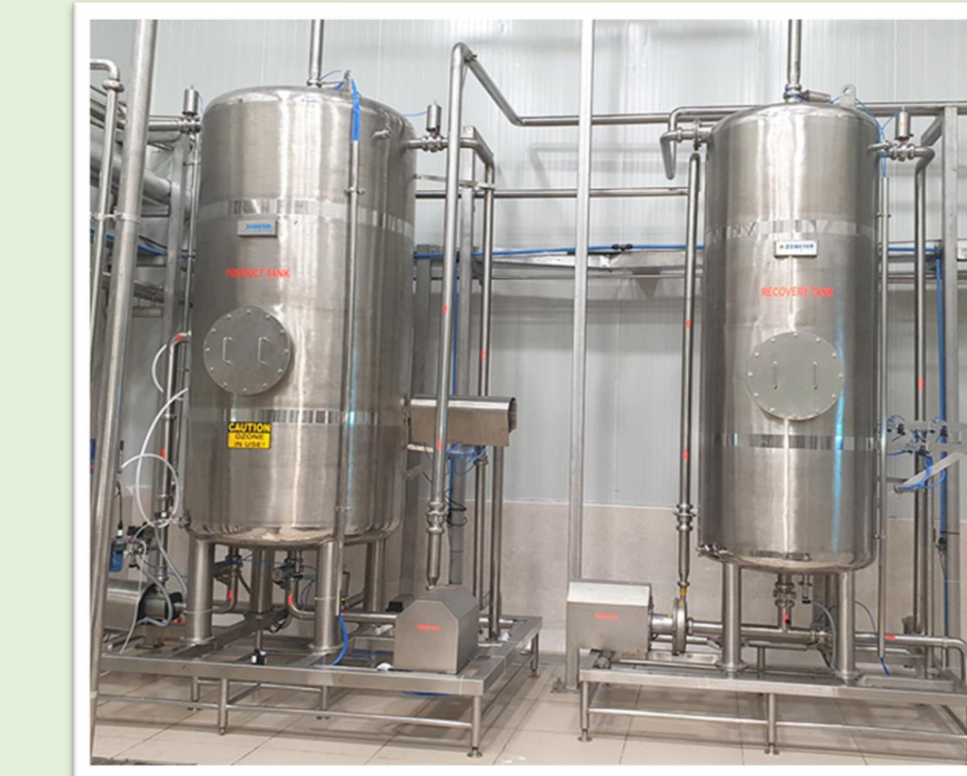
Figure: Ozone Contact Tanks
