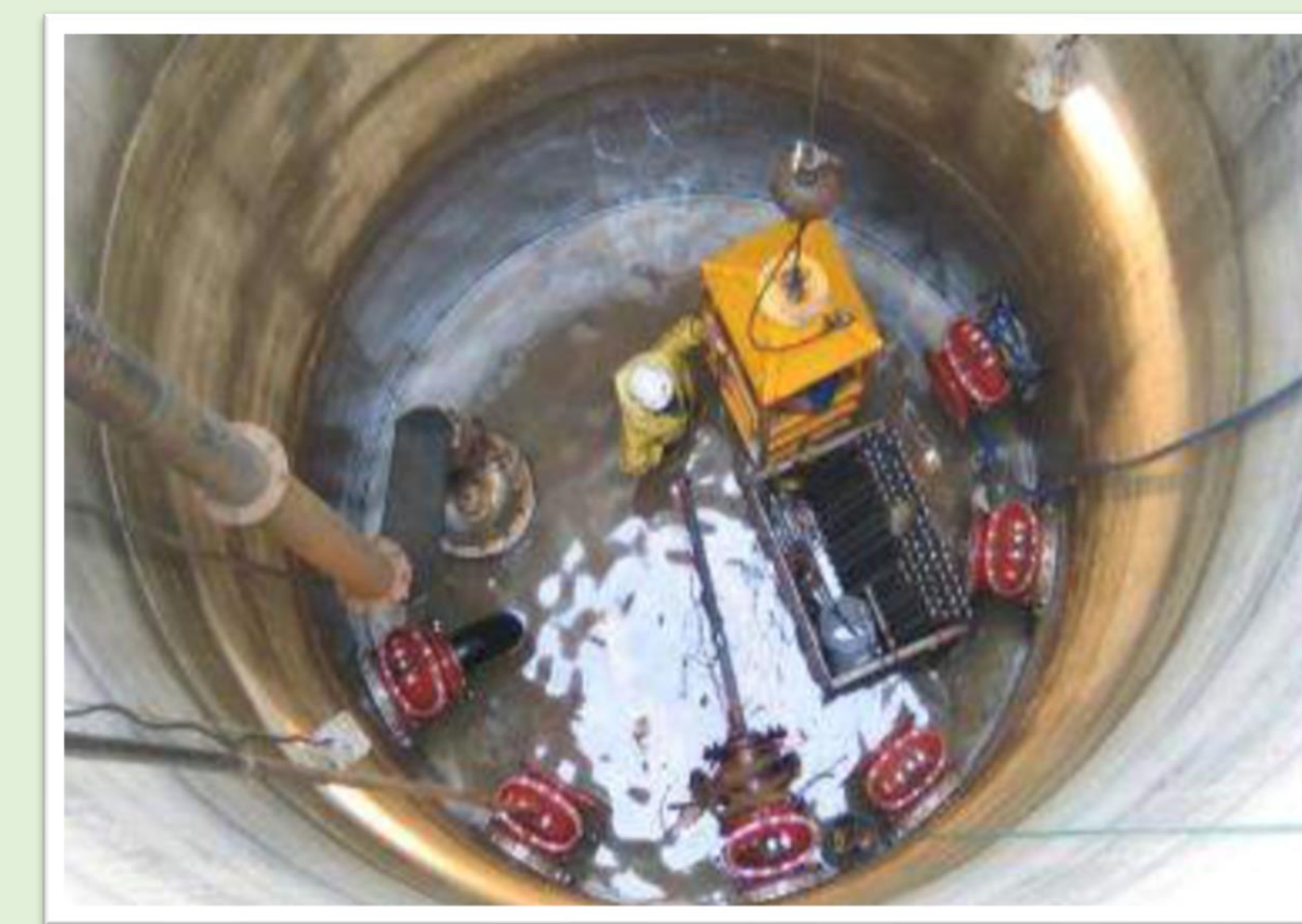
Figure: Inside The Radial Collector Well
