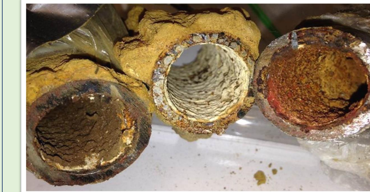
Figure: Corroded Piping
