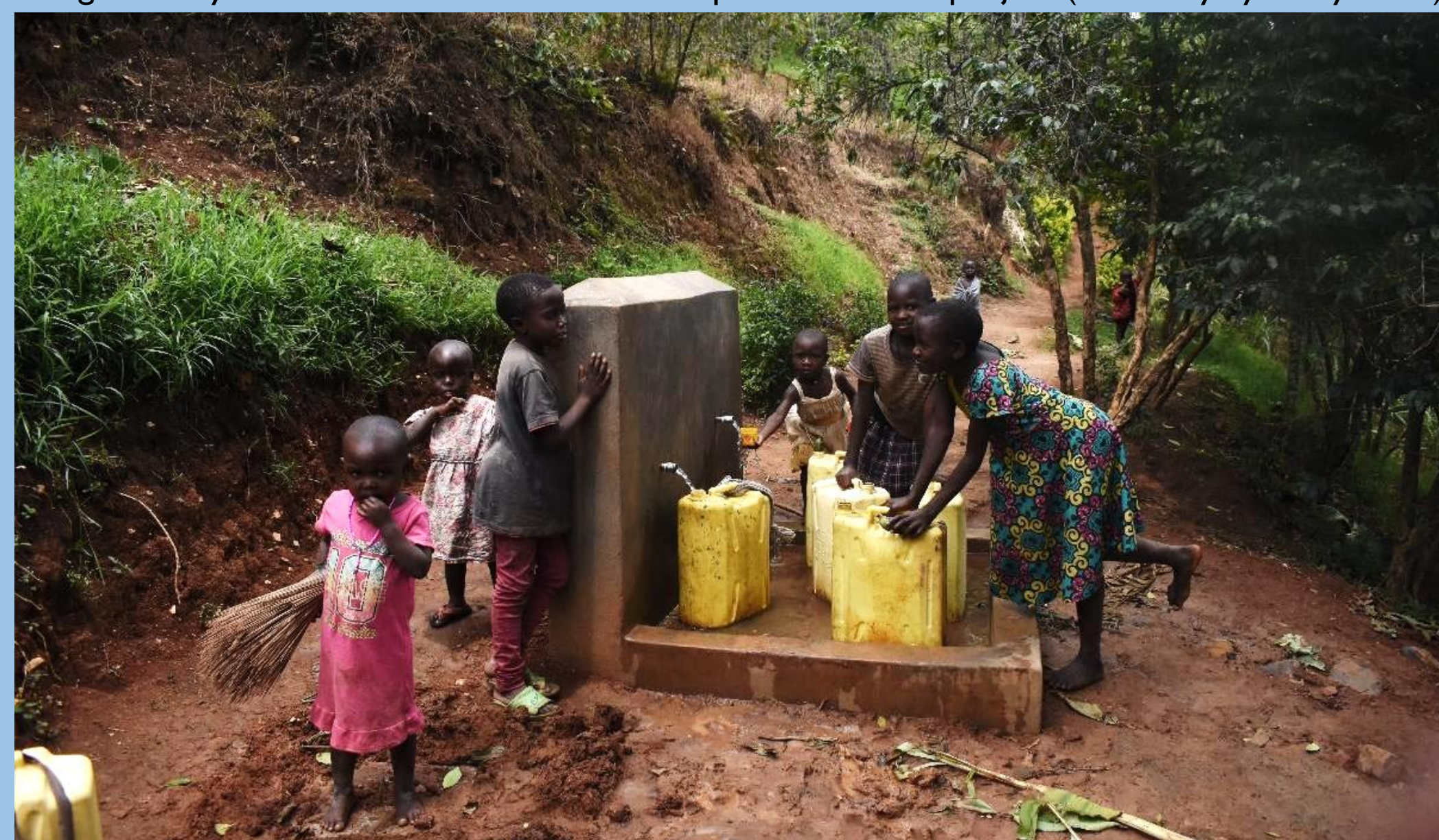
New gravity system; the project was affected by COVID and flooding (Courtesy Lydia Kyokaali)
